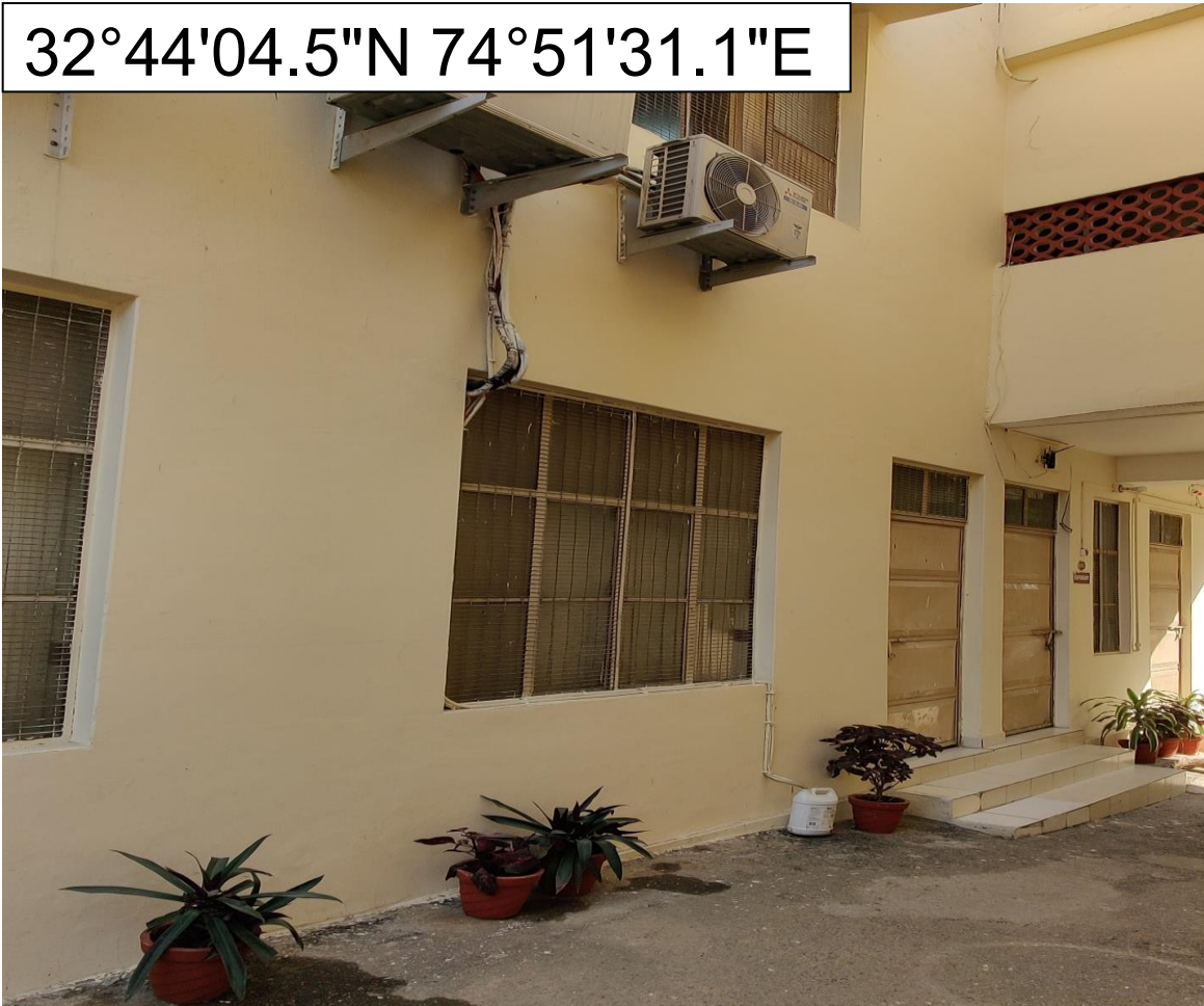
Waste Water from AC Being Collected in Container
